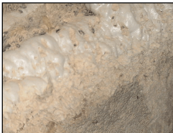
Figure 10. Bird and beetle damage where the crack between the concrete stem wall and plate was sealed using 2 lb/ft 3 foam.
