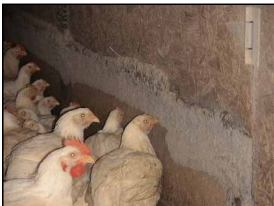
Figure 6. Bird damage to 2 lb/ft 3 polyurethane insulation
