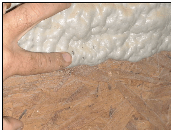
Figure 9. Small holes caused by darkling beetles.
